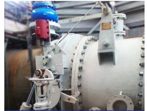
Installation of refurbished 72" butterfly valve and new anti-vacuum air valve for Dolgarrog
