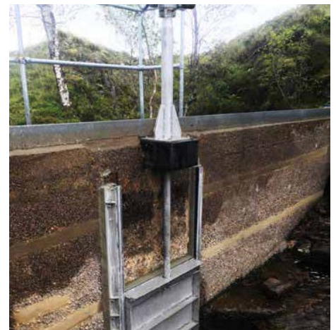
New penstock with floor pillar gearbox & actuator
