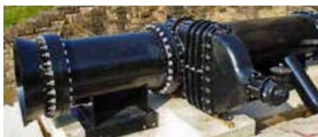
Reservoir spec gate valve - final installation
