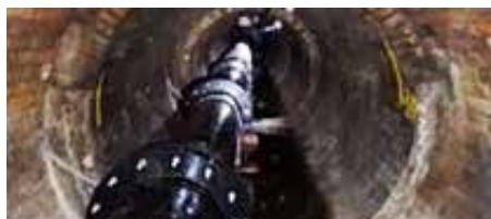
Original upstream 450mm diameter pipework
